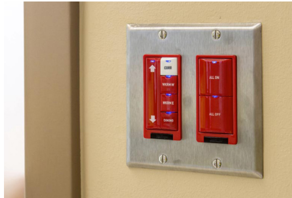
Evaluators at Parkland Hospital recommended engraved switch buttons for simple, intuitive lighting control rather than touch screens
